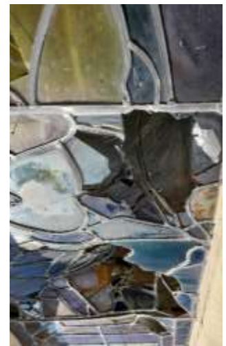
One of the damaged panes
